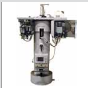
Valve manifold & electronic controls
